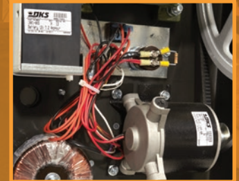
DC Motor & Battery Backup for continued gate operation if AC power is lost
